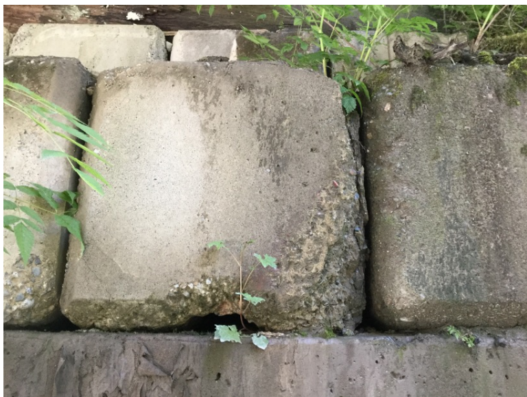
Lock block condition at right bank abutment
