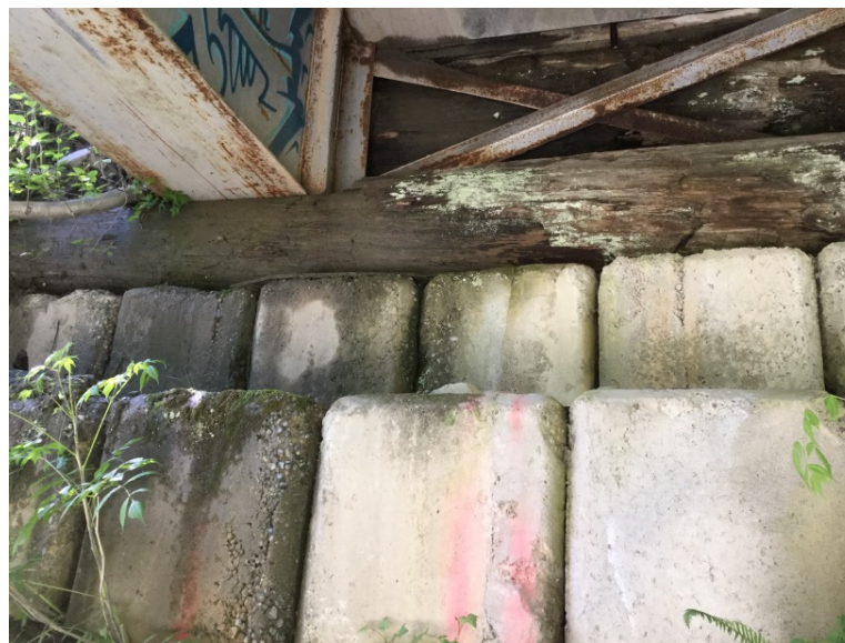
Lock block condition at right bank abutment
