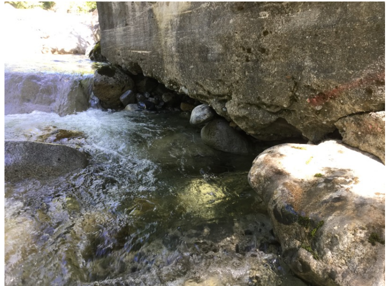
Scour under upstream left bank CIP
