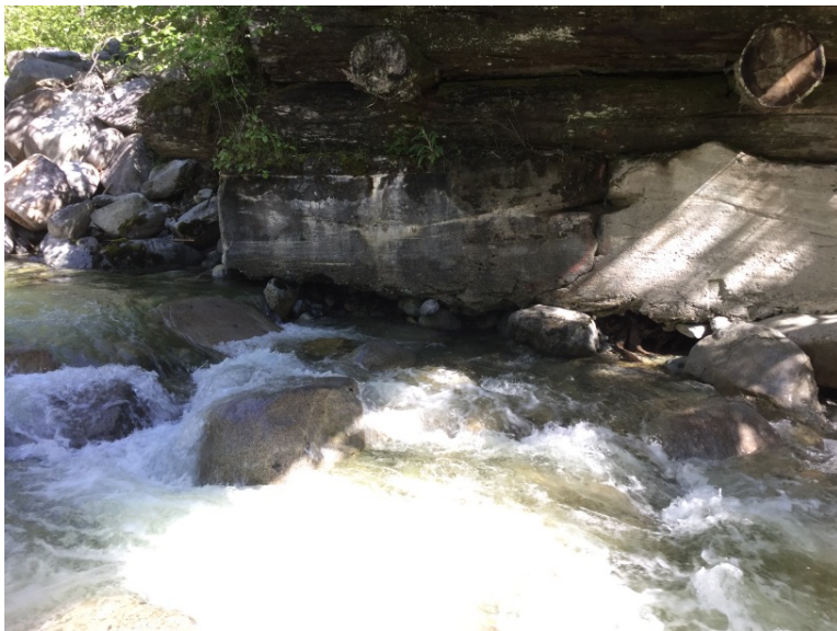
Scour under upstream left CIP
