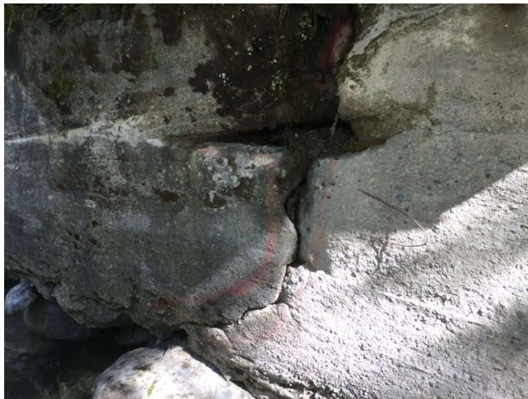
Vertical crack in CIP directly under upstream girder
